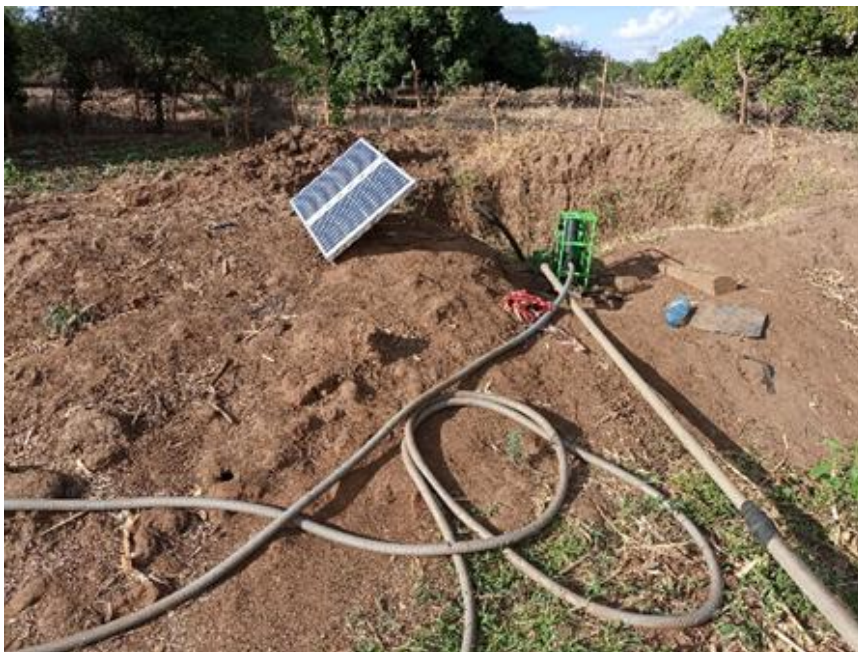
Figure 5: A potable solar powered water pump donated by caritas Kitui in partnership with Brooke EA to support irrigation of vegetable growing
